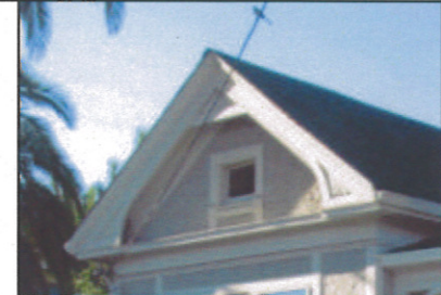
Corbels and other decorative supports can be used to detail roof overhangs.
