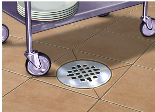
Sanitary Sewer Drain: An indoor drain that flows to the sewage treatment plant.
